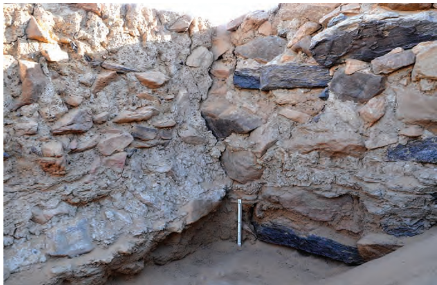
Figure 11 / Elevation of the enclosure wall on the right and of an inner structure wall on the left (area 3). The foundations of the enclosure wall appear to be only of 20 centimetres deep.
